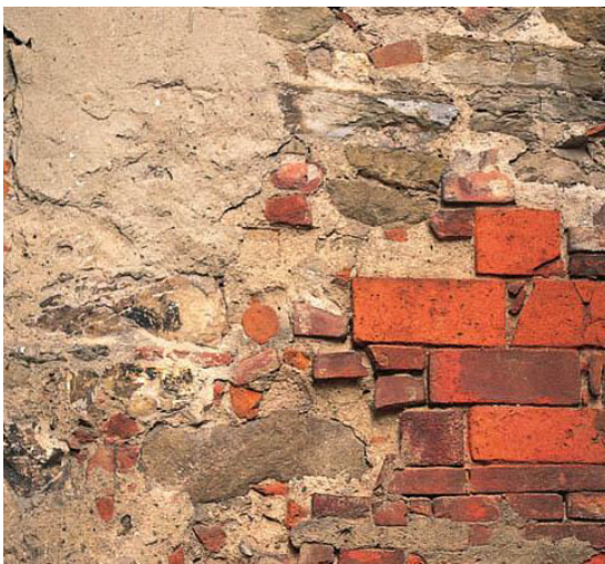
Image 29. Erratically repaired brick wall
