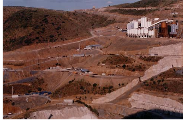
Figure 7. Part of the massive Côa dam construction site in June 1995, at the time it was abandoned.
